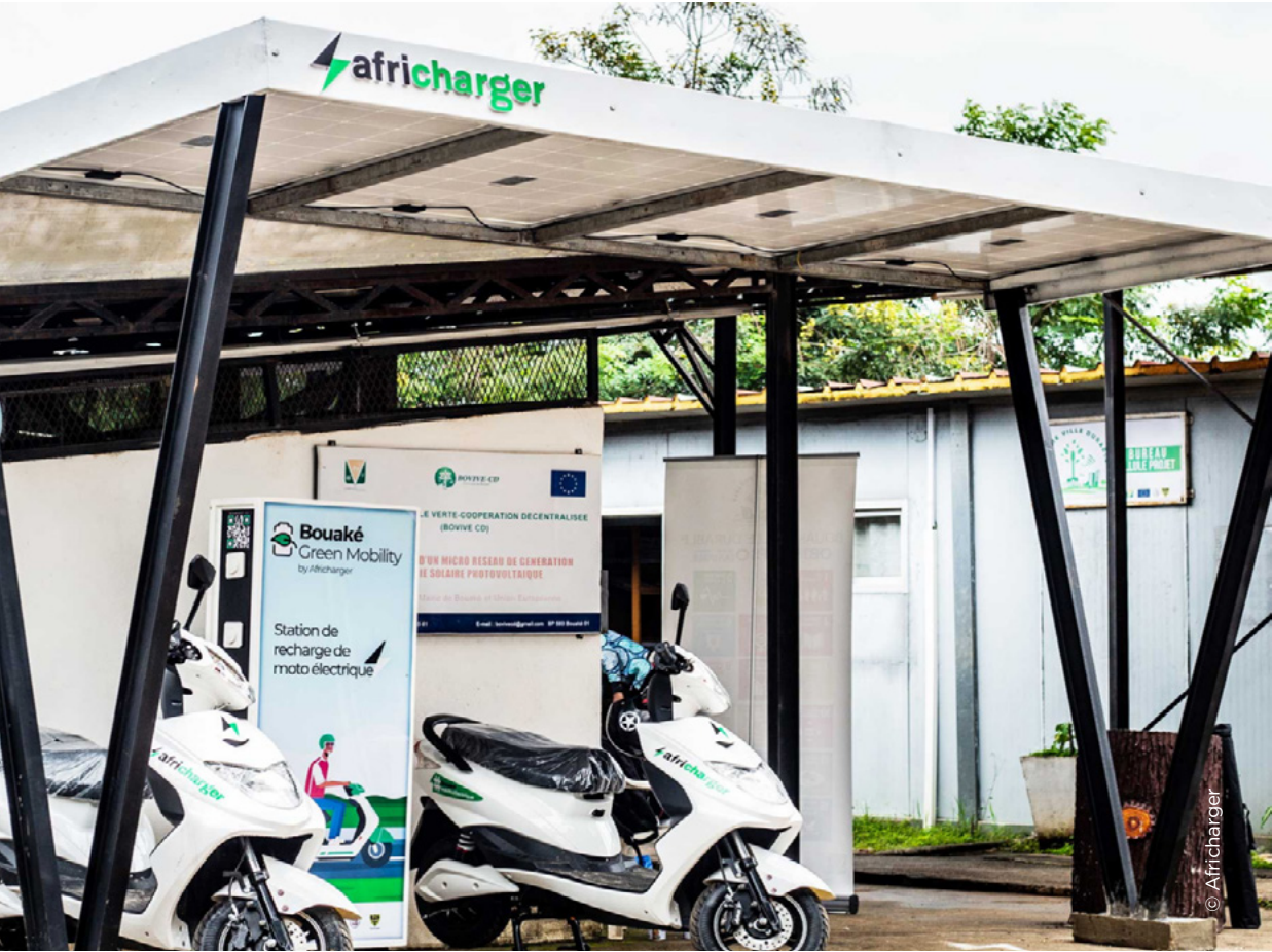
Image 44 : First solar-powered electric motorcycle charging station in Bouaké.
